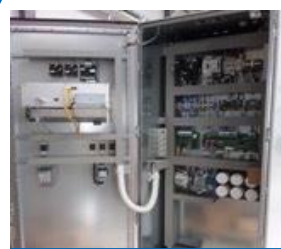
Power Converters for the entire facility
