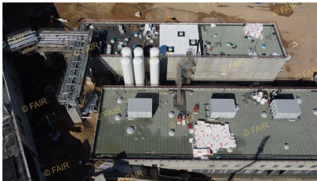
HE- Tanks – Filled with Helium for Cryo Commissioning
