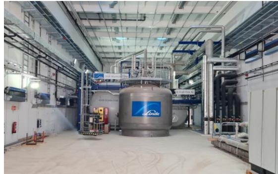
Cryo 2 ready for Commissioning
